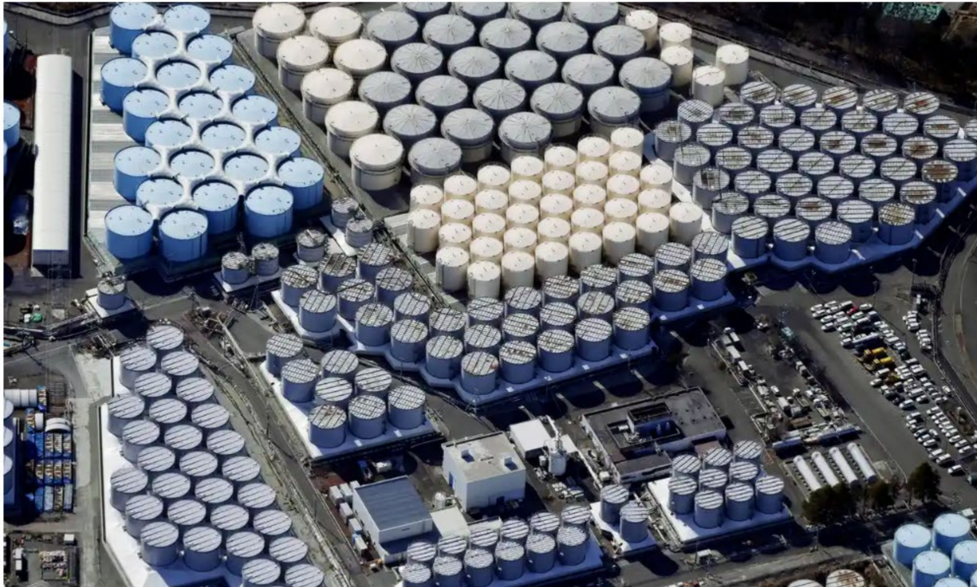
📷 An aerial view shows some of the storage tanks for treated water at the tsunami-crippled Fukushima Daiichi nuclear power plant. Photograph: Kyodo/Reuters
