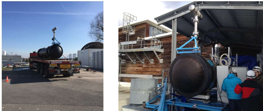
Fig 3.8: Installation of the condenser of the ATLAS thermosiphon on the roof of the CERN LHC Point 1 facilities building (15 meters above ground level, 92 meters above the ATLAS experimental cavern).
