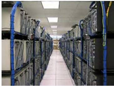
Data centers: Temperature measurement
