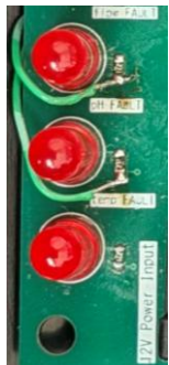
Flow Fault LED
