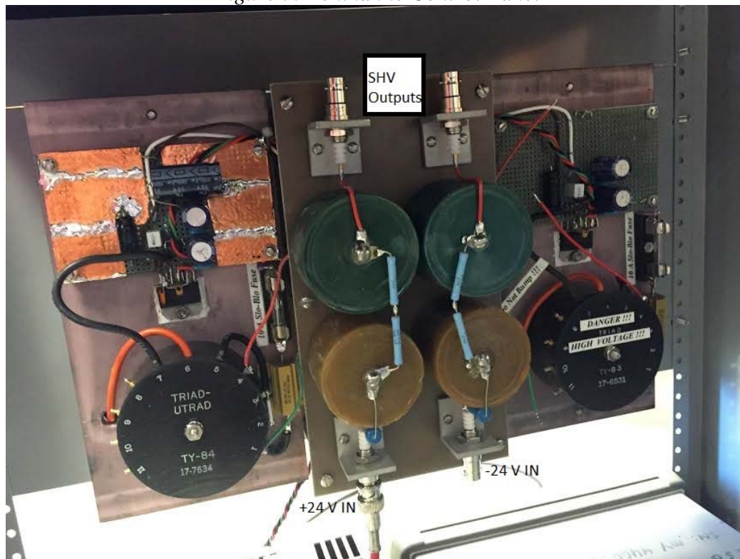
Figure 5: Behind the Control Panel
